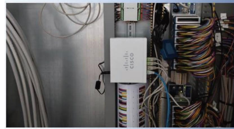
FIGURE 9: Card cabling in the DAS frame.
