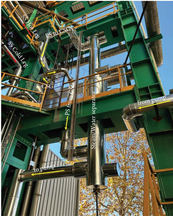
FIGURE 3: View of primary side of ELSMOR plant and S-CSG.
